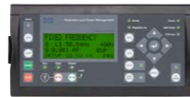
PPM-3 Protection & power management system.
